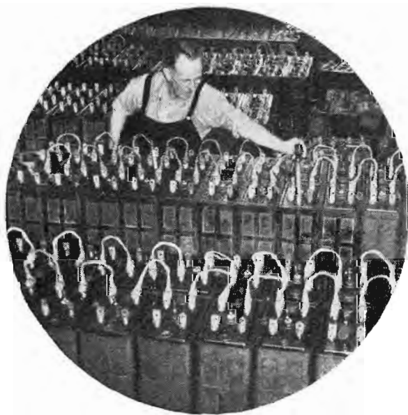
Battery charging is big business.
